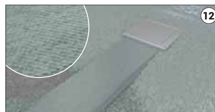
12 Then, apply another thin layer of cement mortar on the mesh wire.
