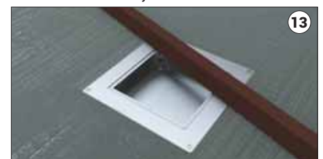
13 Apply the regular screed on top and use a gauge to level based on a pre-laid rope.
